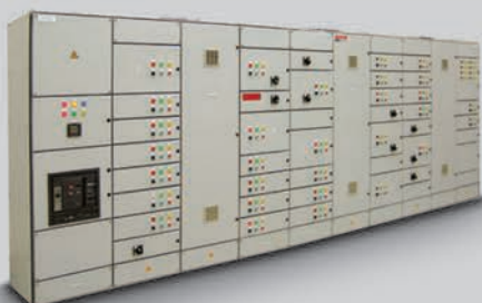
WITH DRAWABLE LV SWITCHGEAR
